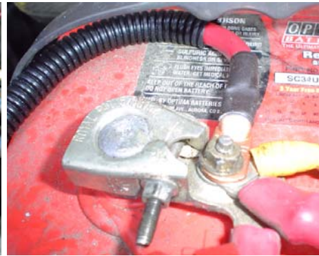
Positive battery conxn from ANL fuse block.
