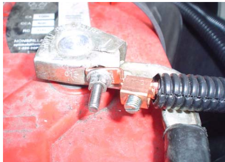
Ground conxn from Quicktifier.
