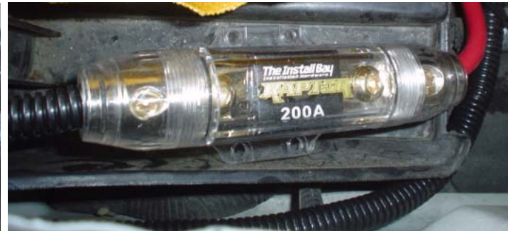
200 amp ANL fuse block between Quicktifier and Battery (driver side).
